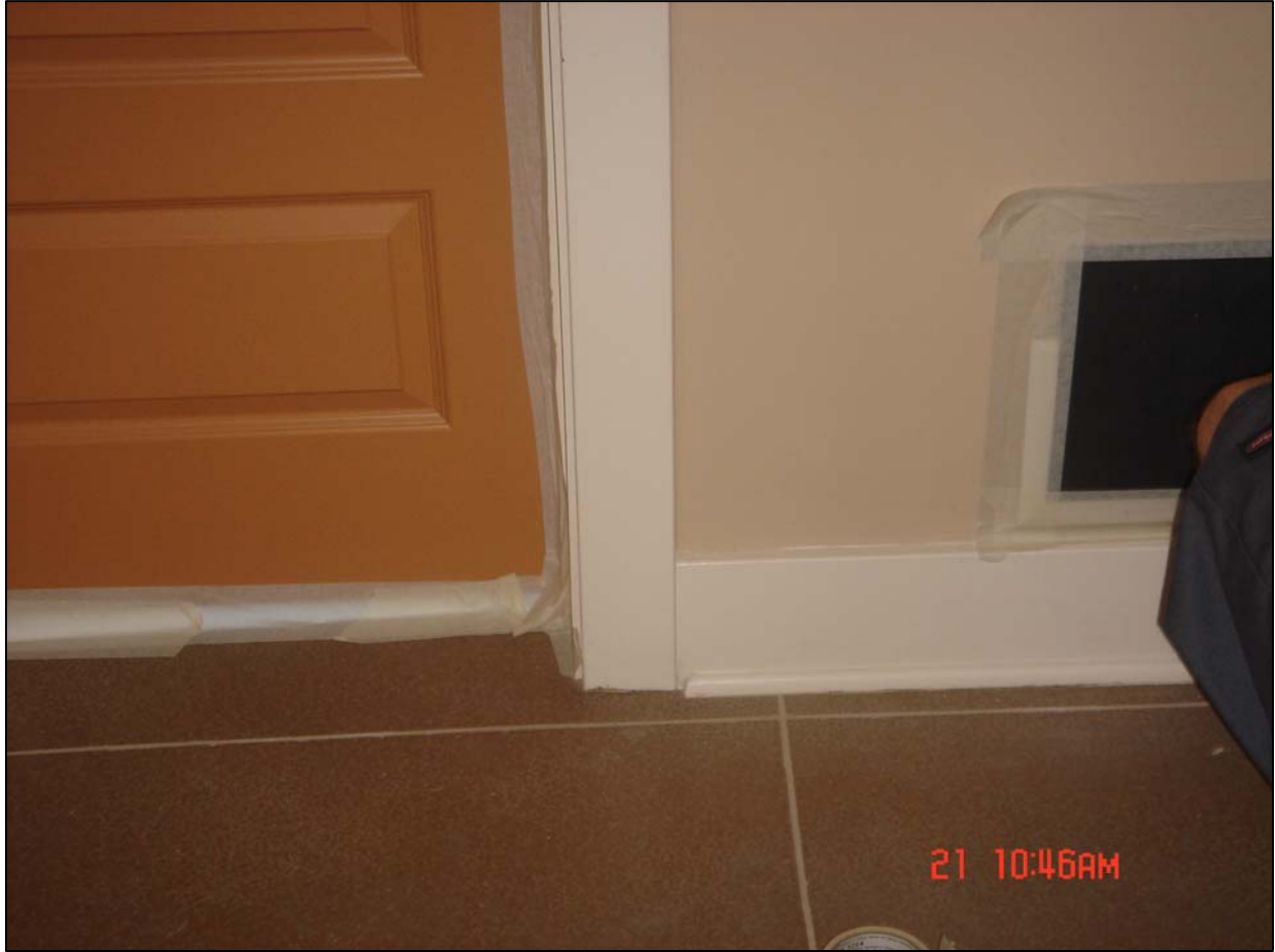
Figure 9: Floor to Wall Infiltration Gap
