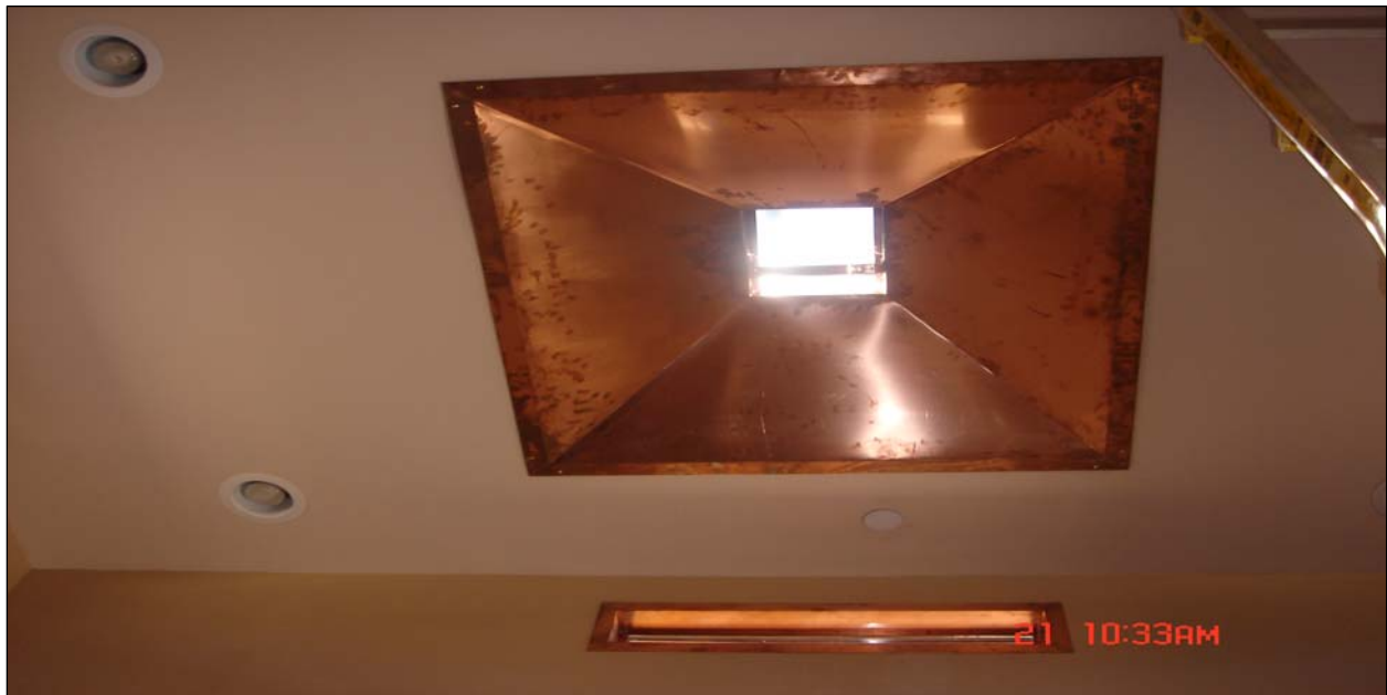
Figure 7: Example Custom, Site Built Skylight Penetrations
